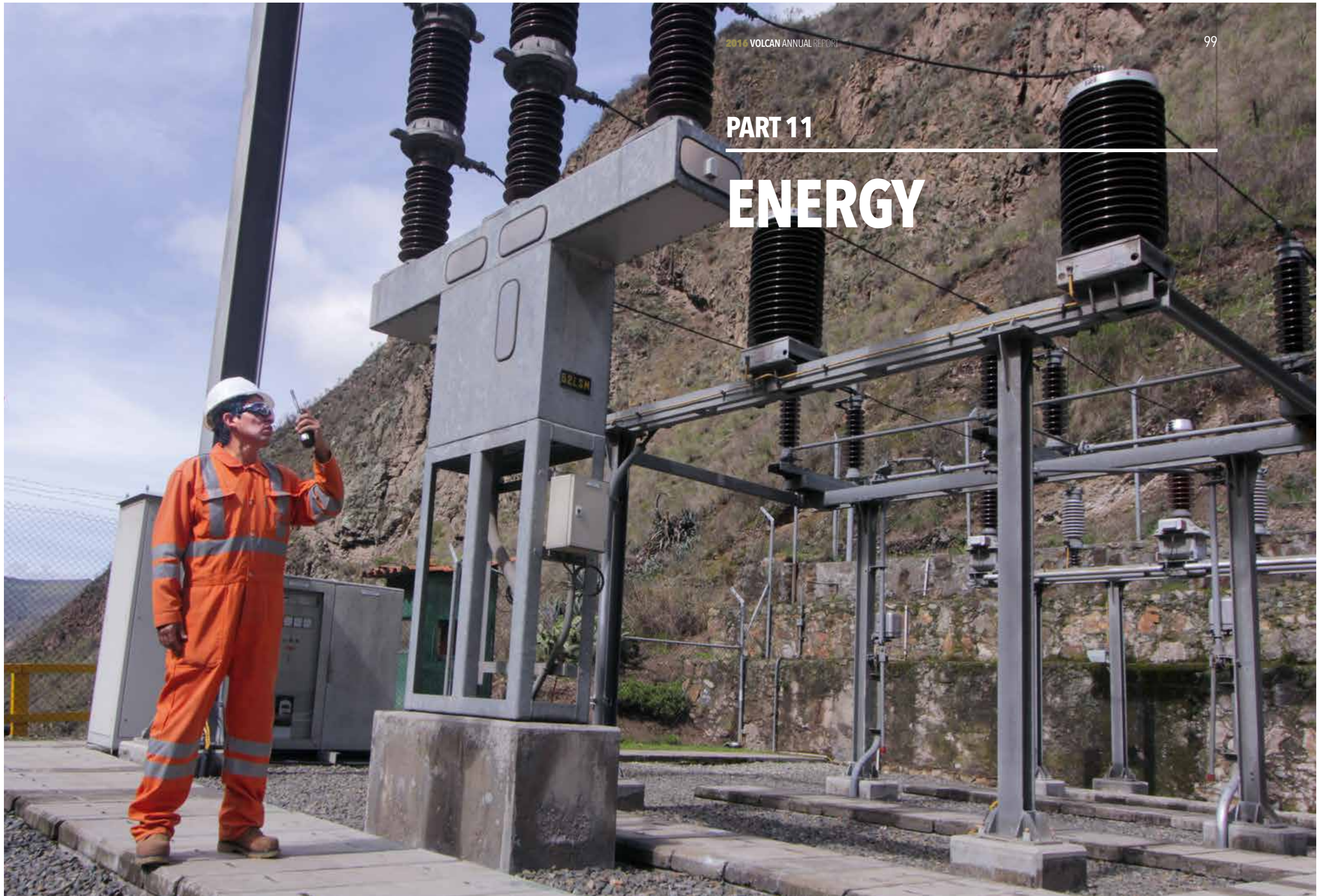
San Mateo substation - Huanchor Hydroelectric Plant
