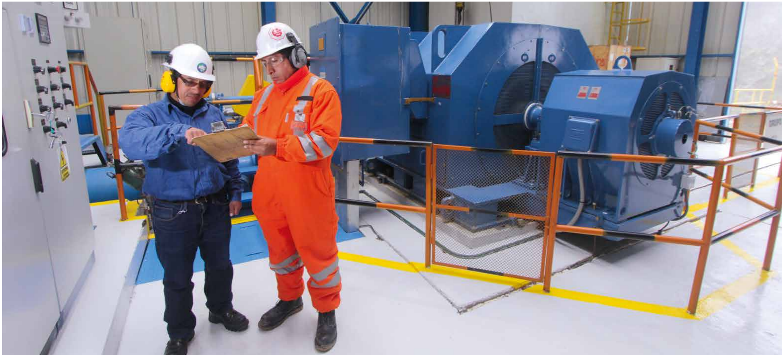
Powerhouse - Baños IV Hydroelectric Plant
